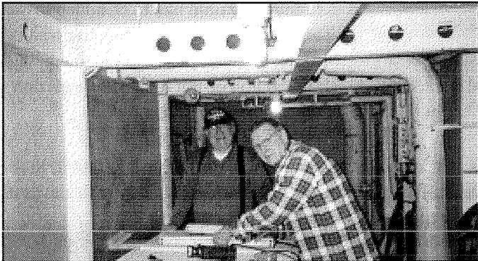
John Hemminger (foreground) and Tom Manning getting ready to make a cut for an access panel.
