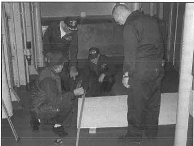
Tom Giardina, Al Nannini, Roland Cote and John Hemminger laying out ceiling panel
