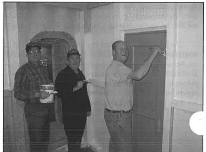
Tom Giardina, Roland Cote and Don Batty priming inside of radar room
