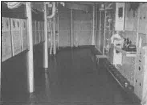
Picture shown here is what the area of the radar room looked like before we started work.
