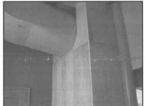
Side and back view of extended radar room going up to overhead.
