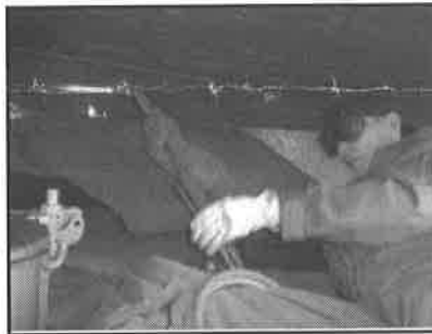
Harry Miller cutting out rusted section of duct that returns under the turret.
