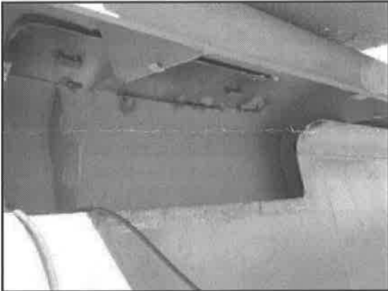
Area that was cut out to be able to get to the damaged section of duct. New piece of plate is tack welded inside of duct..
