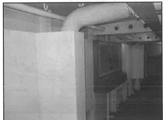
Side view showing boxed in vents.
