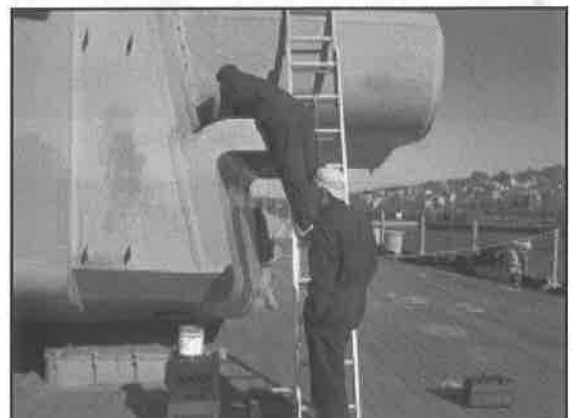
Roland painting top of duct with Harry looking on and footing ladder.
