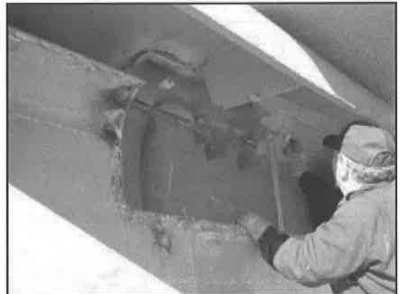
Roland painting new steel. Area is inside the duct. Note new drain line installed in duct.
