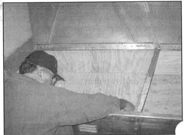
Roland checking the fit of the new shelves and back panel we just installed.
